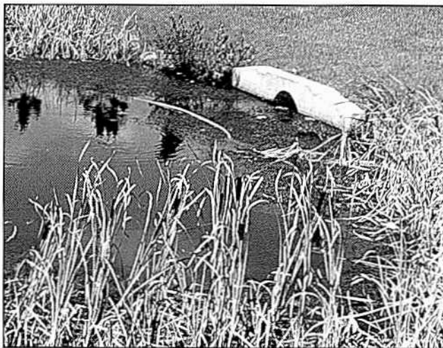
▲ Typical inflow pipe.
